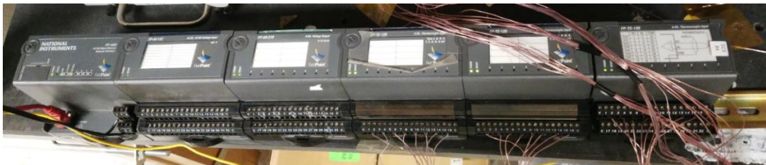
Figure 3.14: NI field point for temperature recording.
