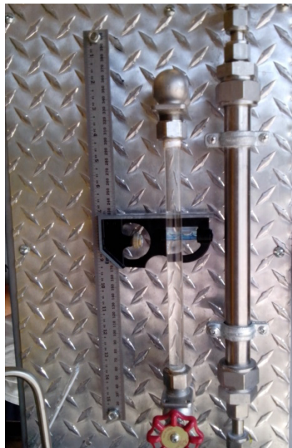
Figure 4.10: Level gauge used as part of flow rate determination method for cooling coil.
