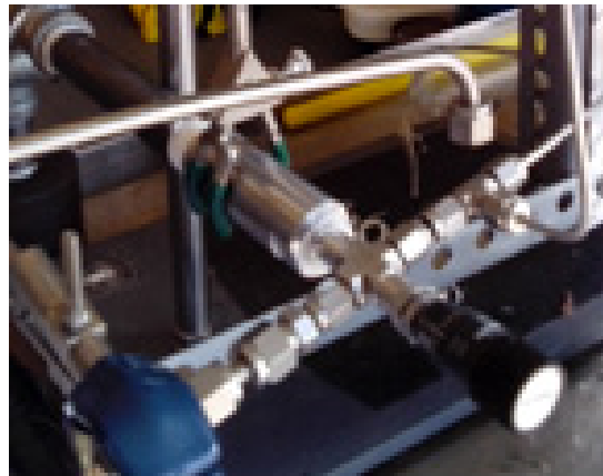
Figure 3.16: Photograph of the ejector as installed in the system.
