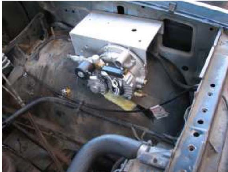
Figure 3.2: TN2 regulator installed parallel to the engine.
